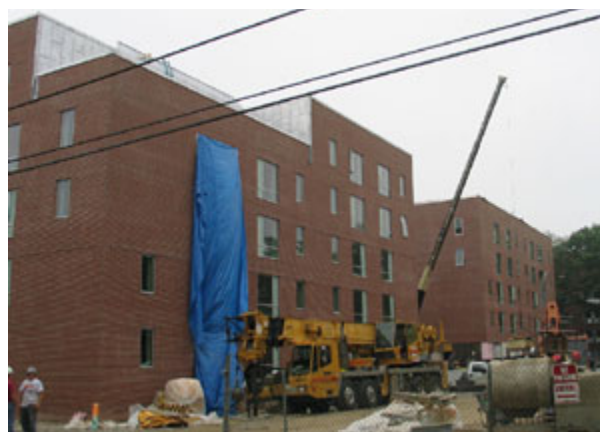
Figure 12: Construction of West Hall, a LEED certified residence hall at Bowdoin (Bowdoin College Sustainable Bowdoin 2005 "LEED Residence Halls").
